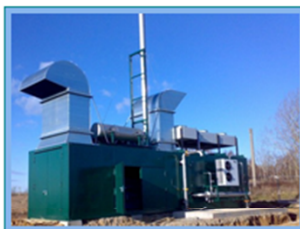
370 kWh biogas CHP cogeneration system
