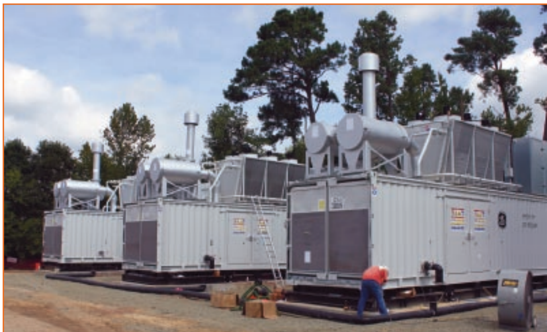
Methane Power's plant in Durham city utilises three GE Fenbacher engines to generate 3.3MW of electricity
