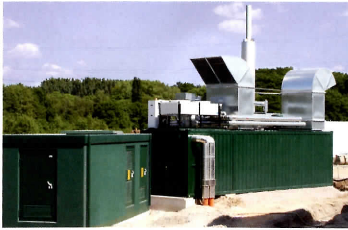
The new CHP plant, provided by 2G Cenergy, will produce electricity and thermal power
