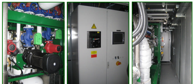
Inside View, complete and "connection-ready" The 2G ® CHP Cogeneration Module
